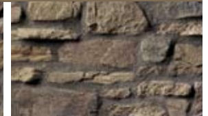
Wide Mortar Joints, Overgrouted, Horizontal Placement
