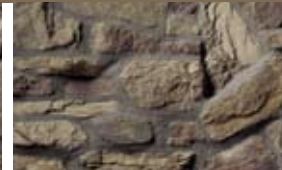
Wide Mortar Joints, Overgrouted
